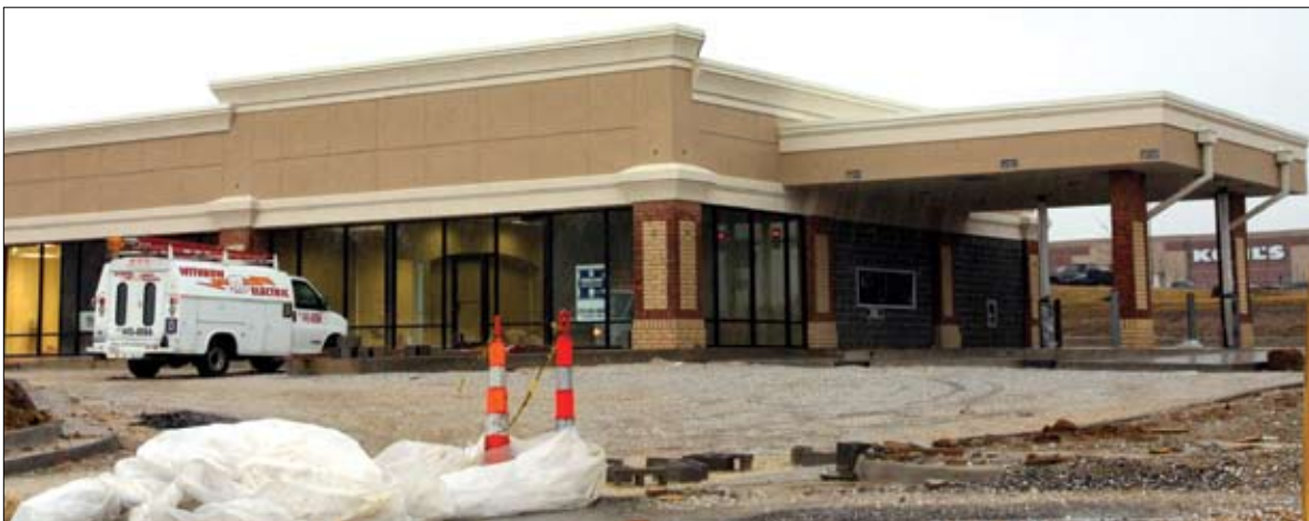
River Region Credit Union and Sports Clips, a franchise owned by Jeff and Kim Guinn, will move into this 7,200-square-foot building on the southwest corner of Grindstone Plaza, which builder Jeff Herigon of Hercon Construction plans to finish this spring for the owner, THF Realty, at a cost of about $1 million.
